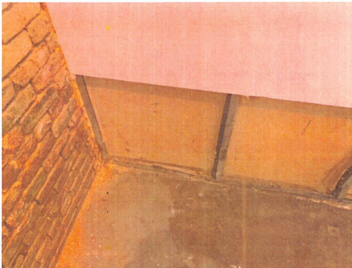
Inside the living room area wall cavity – tape lifts revealed light mold growth is present
