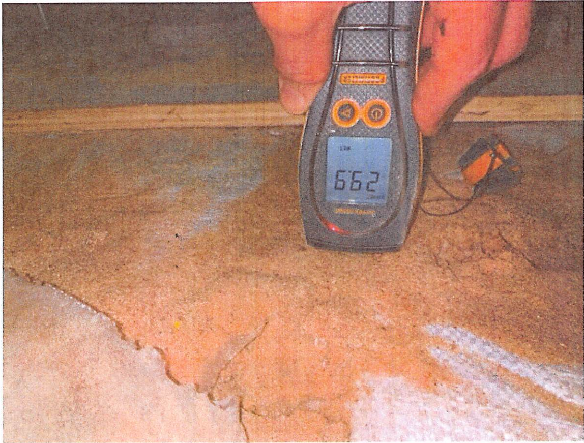
The sand is wet under the raised floor
