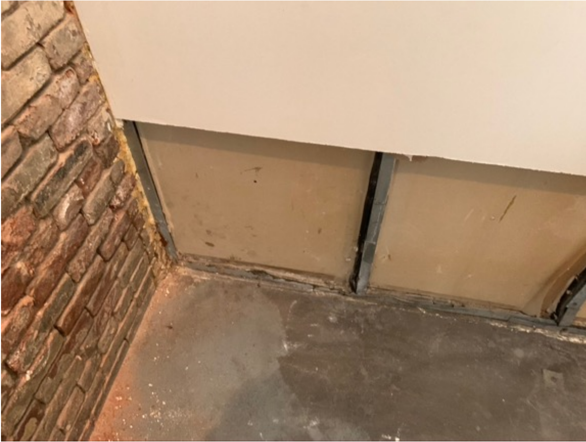
Inside the living room area wall cavity – tape lifts revealed light mold growth is present
