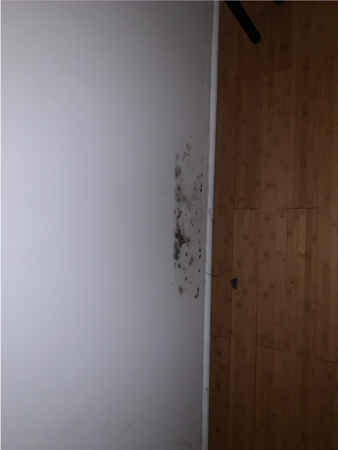
Visible mold on the base of the wall in studio area
