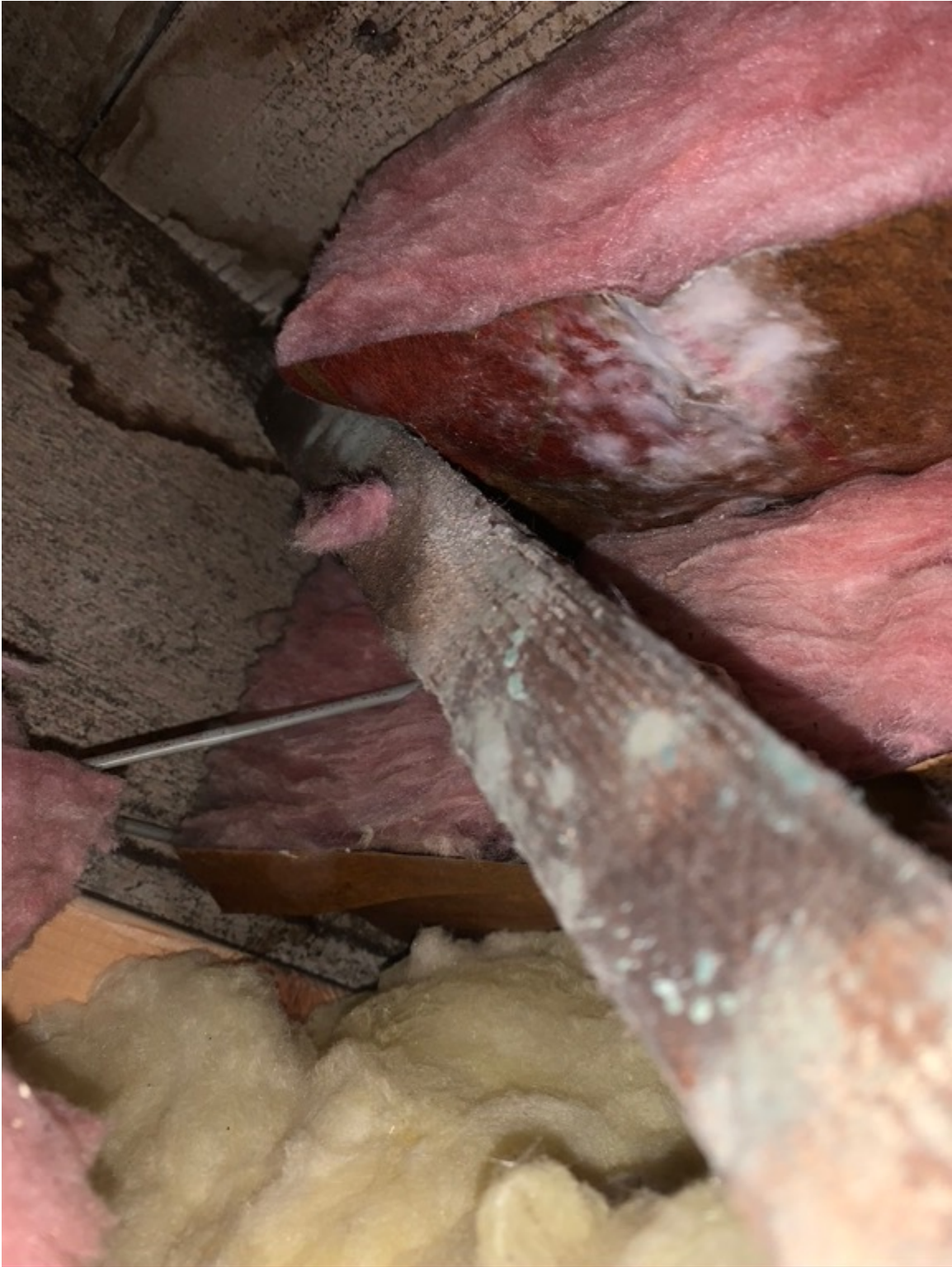
Mold growth on insulation and wood joists on the underside of the floor above
