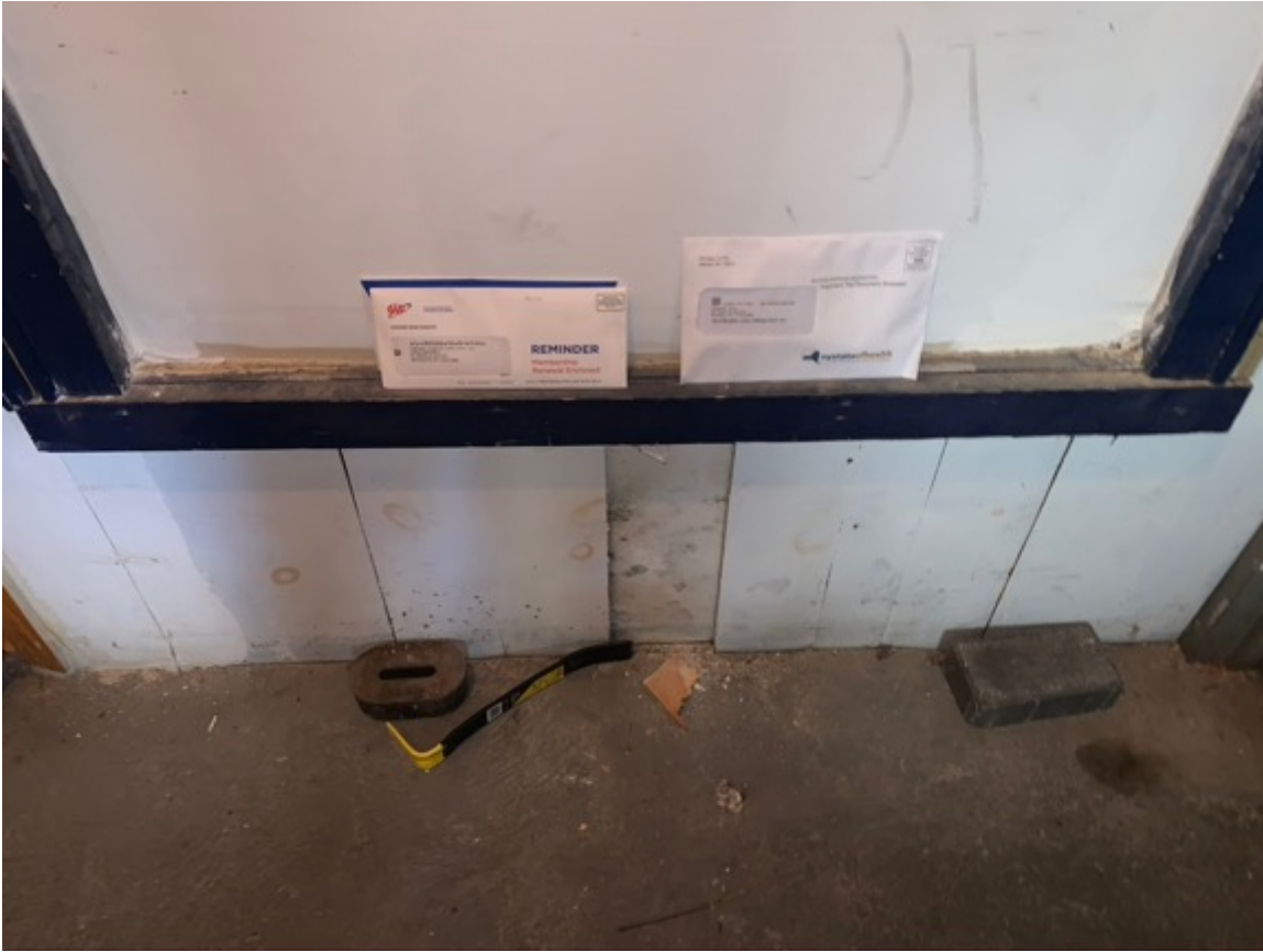
Visible mold behind the removed wood wainscot
