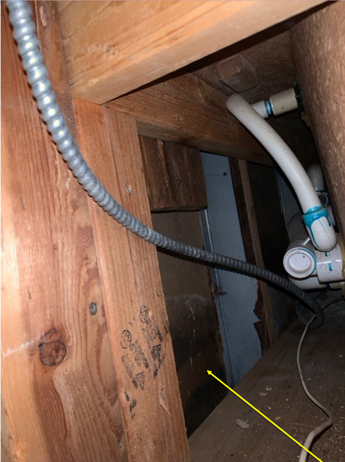
There is water staining and mold growth on the bathroom wall shared with the kitchen.
