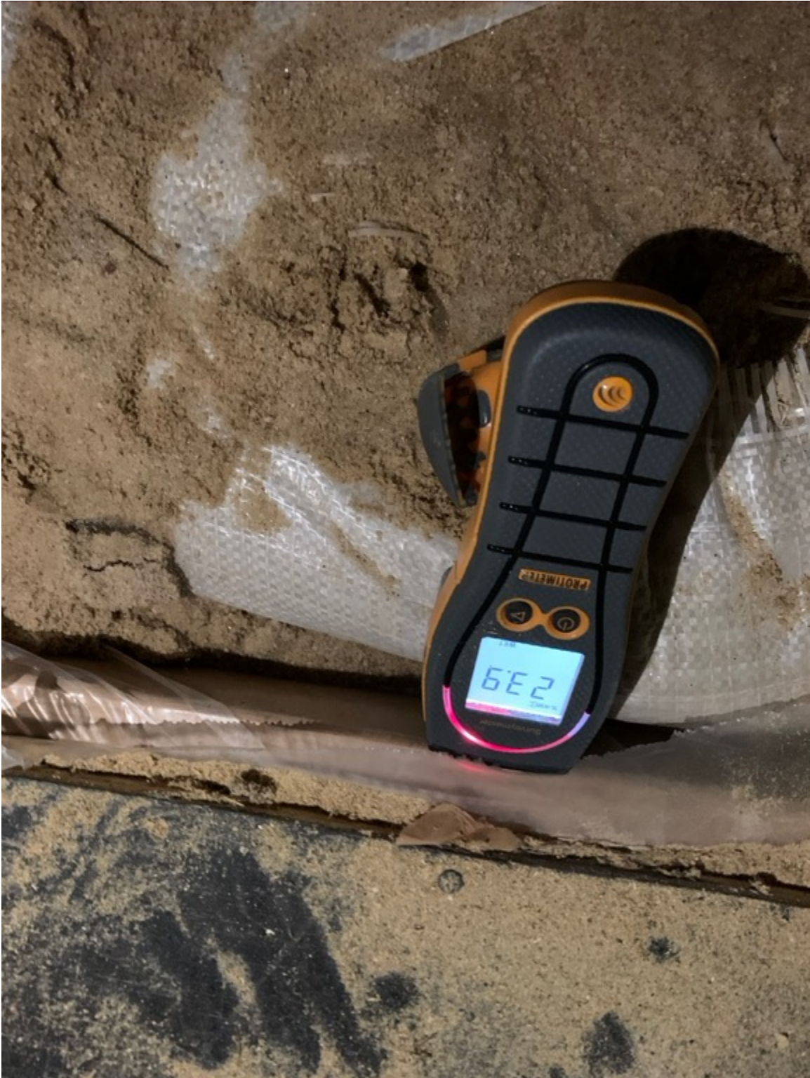
The wood joists adjacent to the sand is wet
