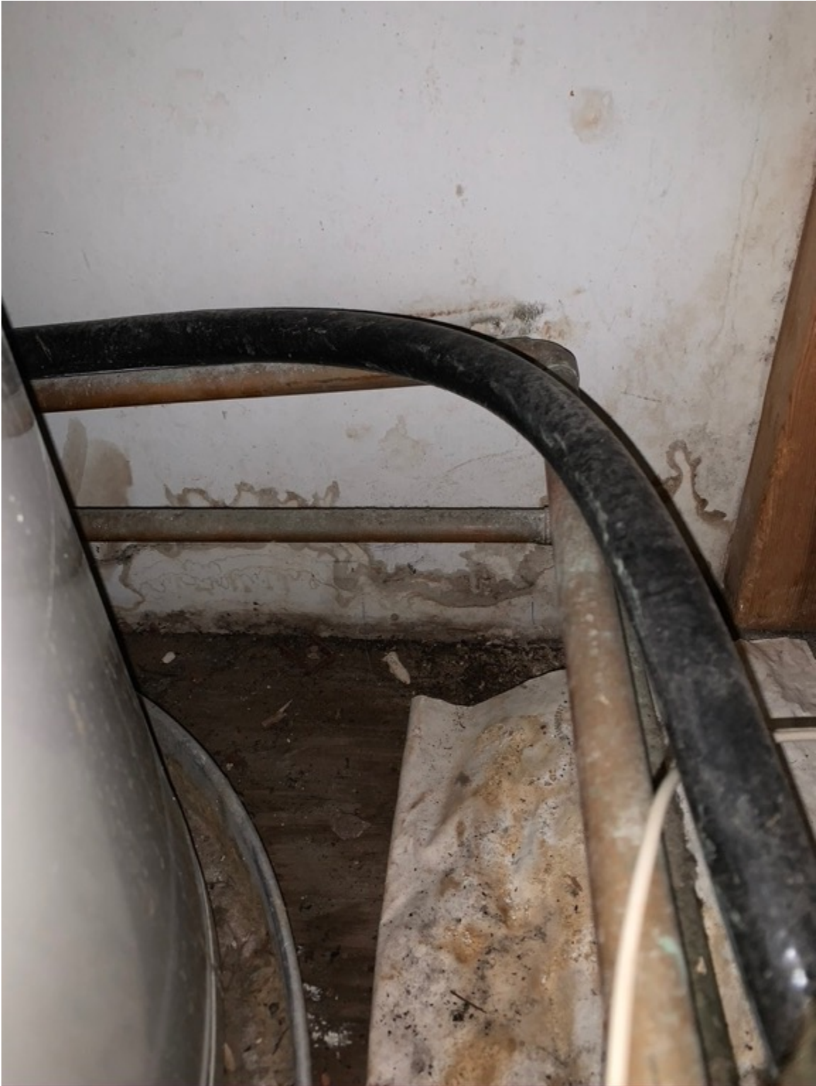
The hot water tank next to the bathtub – there is mold growth on the raised wood floor and on the wall shared with the kitchen
