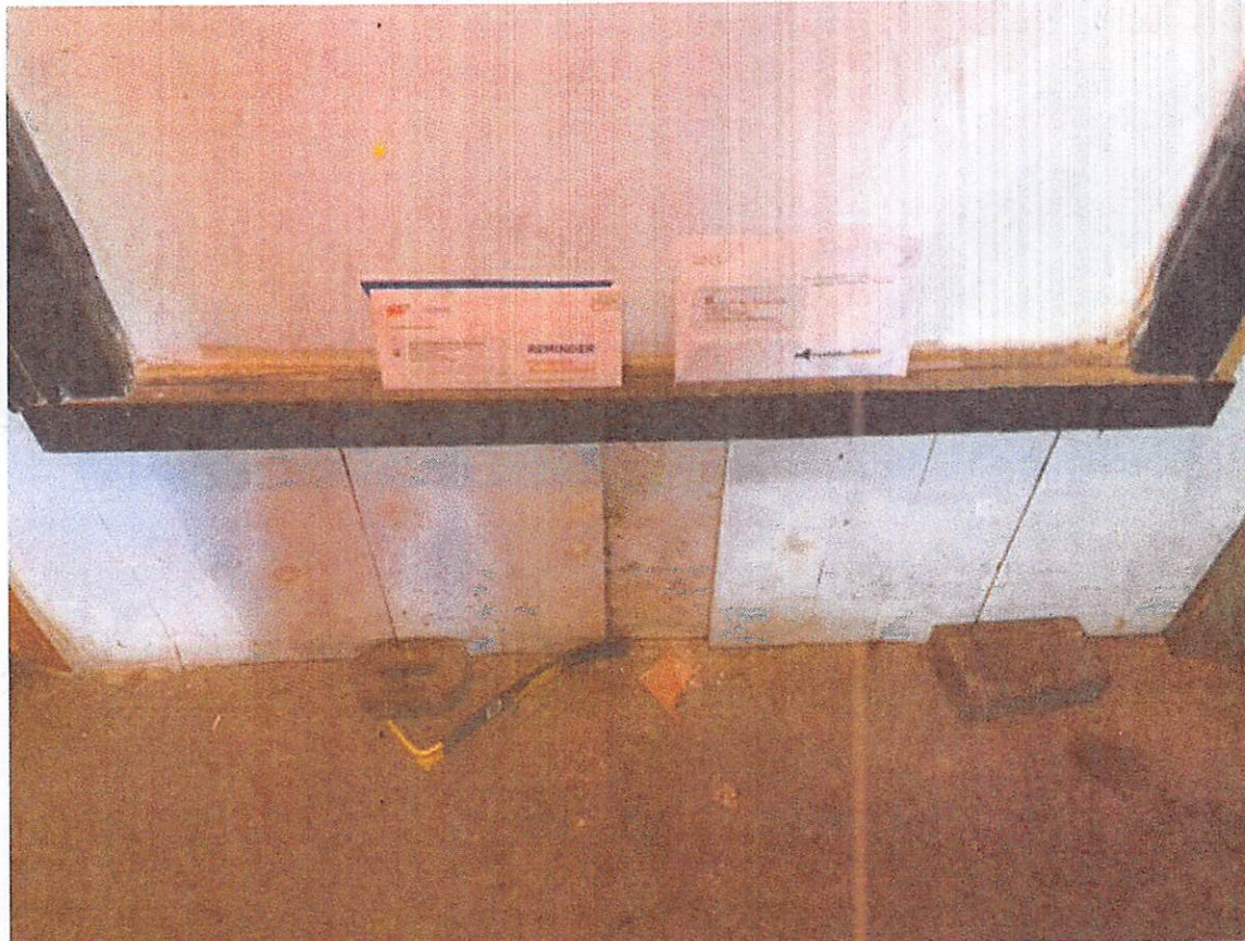
Visible mold behind the removed wood wainscot
