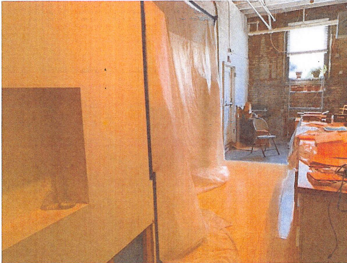
Kitchen area – there is mold growth under the wood flooring
